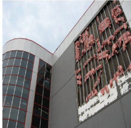
Damage to the Science Center
